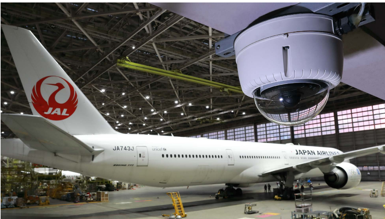
Canon network cameras are installed in the JAL hanger at Haneda Airport
