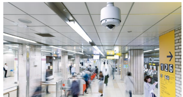
Network camera operating in a subway station
