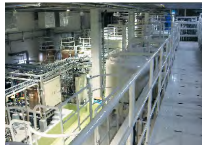
New wastewater processing system (Hiratsuka Development Center)
