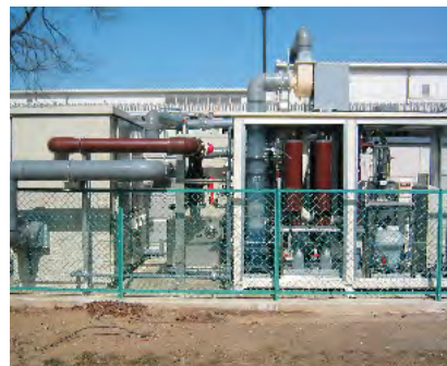
Gas processing-type test equipment for photo-activated water processing
