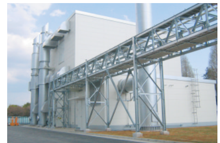
External view of cogeneration system (Canon Chemicals, Iwama Site)
