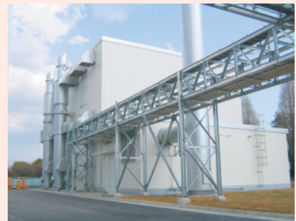
Oita Canon Materials Inc. and Canon Chemicals Inc. have installed cogeneration systems that produce both electricity and heat from direct fuel combustion
