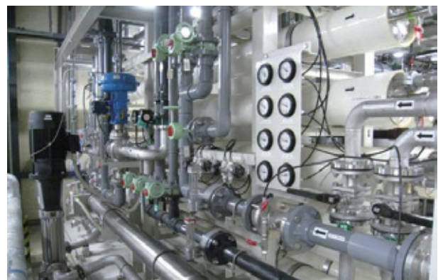
Water purification equipment
