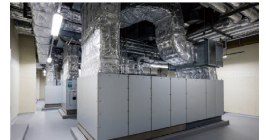
High-efficiency air conditioners upgraded for clean rooms
