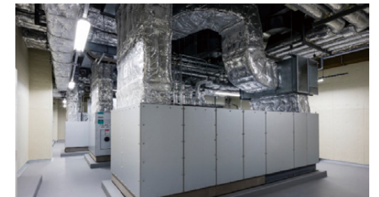
High-efficiency air conditioners upgraded for clean rooms
