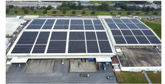
Solar panels installed at Canon Vietnam’s Thang Long Factory
