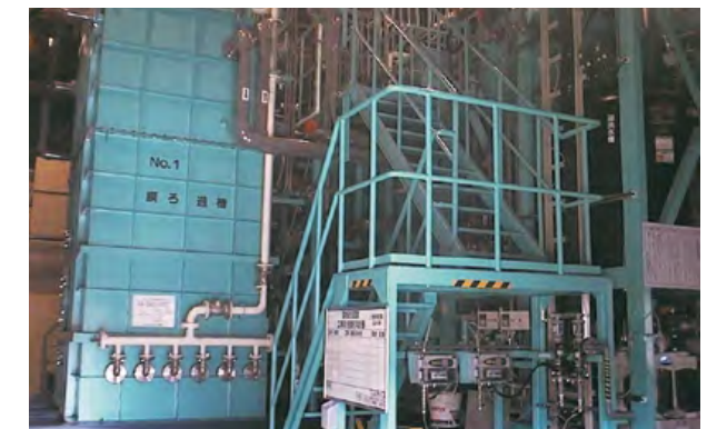
New Closed Wastewater Treatment System (membrane filtration device)
