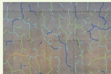
AI-based detection of structural cracks
