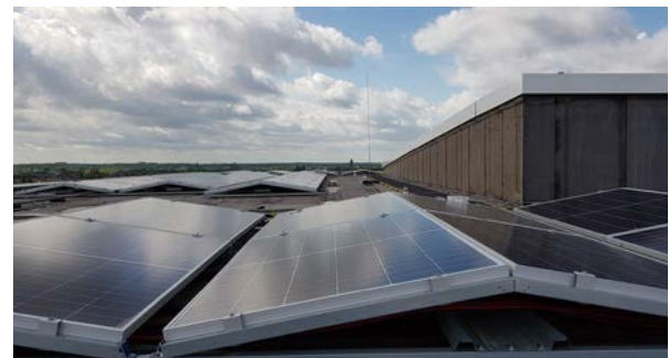
Solar panels at Canon Production Printing Netherlands
