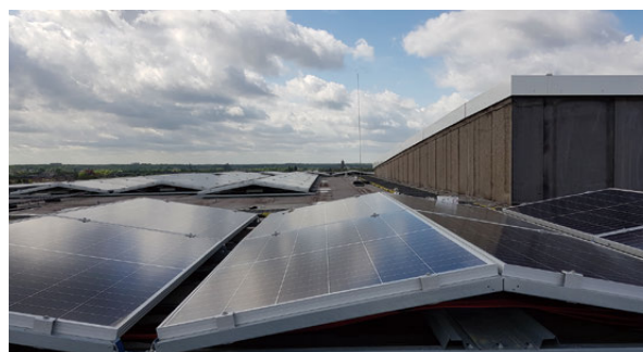
Solar panels at Canon Production Printing Netherlands
